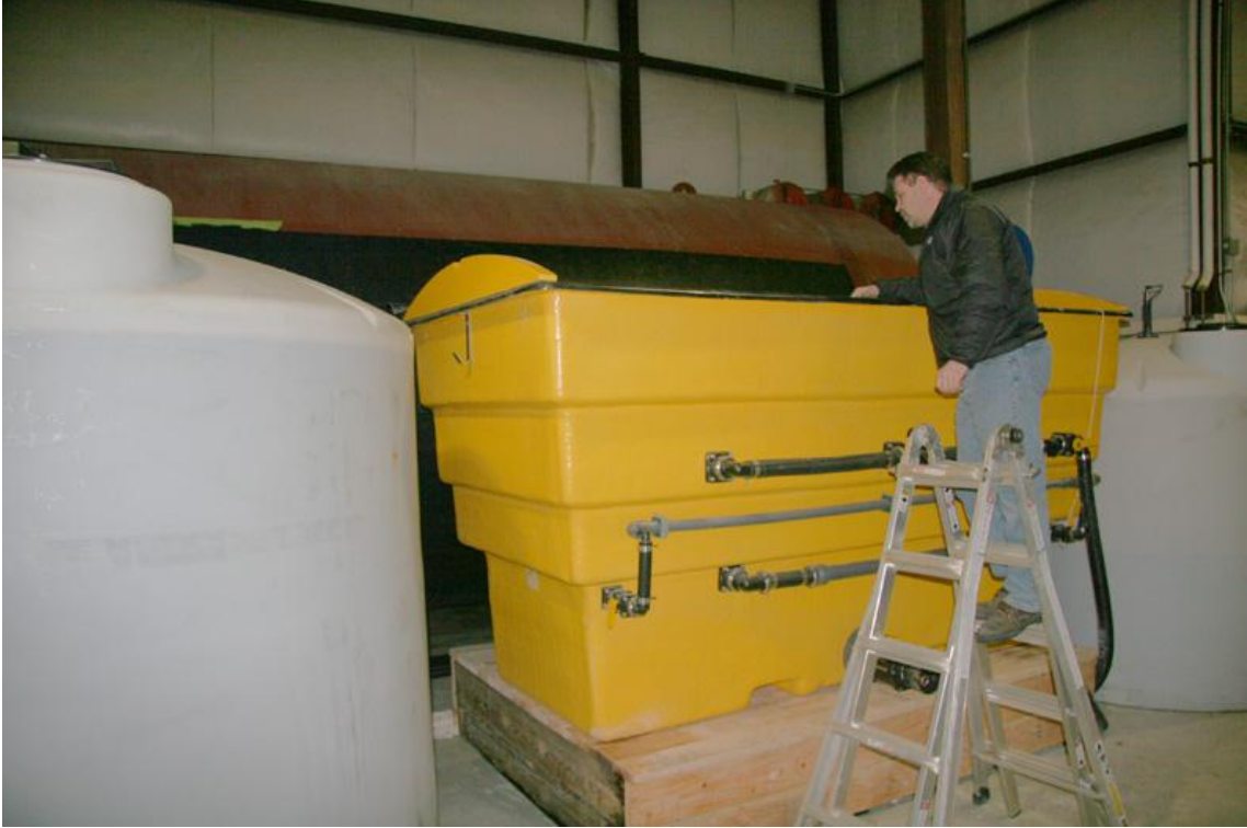
Figure 2 - Salt Brine Mixing Unit and Storage Tank
